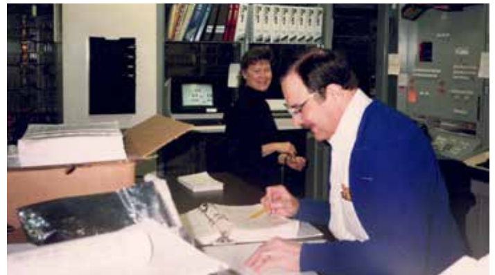
Debbie Nelson and Carl Rudolph in the Minneapolis Downtown Central Office
